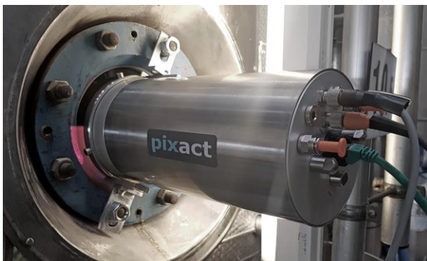
Figure 4. FL installation on the boiling pan sight glass.
